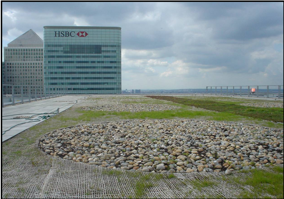
One of Tower Hamlets' many green roofs - Barclays Bank HQ, 1 Churchill Place, E14
